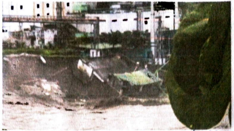
The IRP laboratory was badly affected due to landslide
