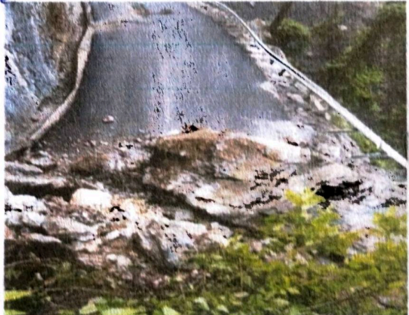
Legship-Nayabazar road was damaged due to Landslides
